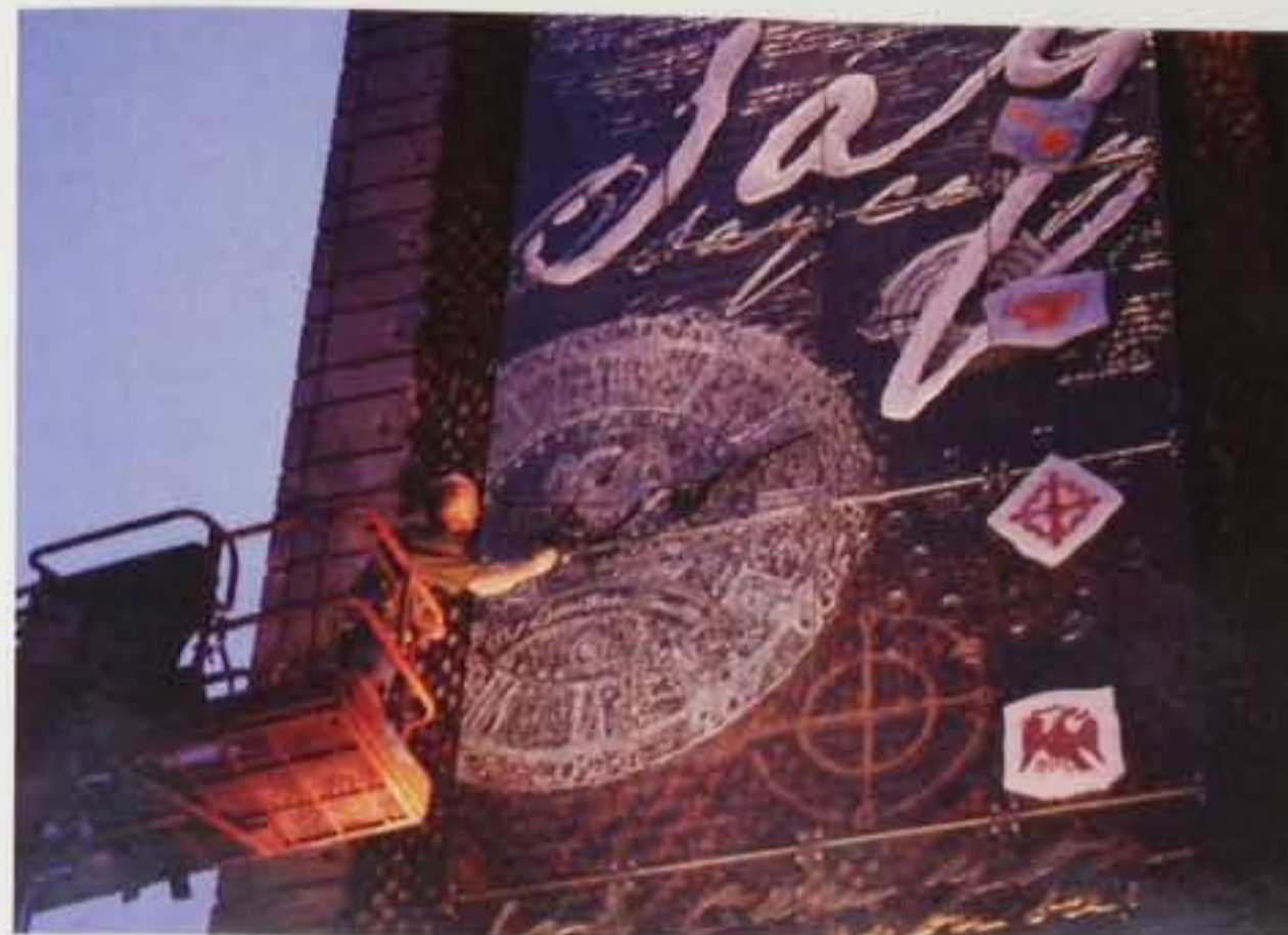
William works on the lift during installation of The Dreaming . The glass was fabricated at Derix Glasstudios in Germany. Photo by Teresa Cochran.
